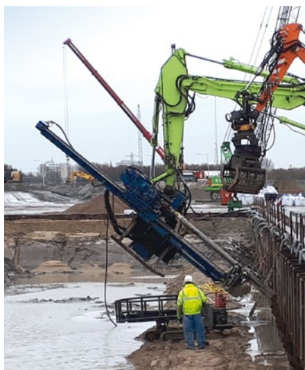
Drilling 178mm casings and 60 m long beneath excavator in sand and gravel
